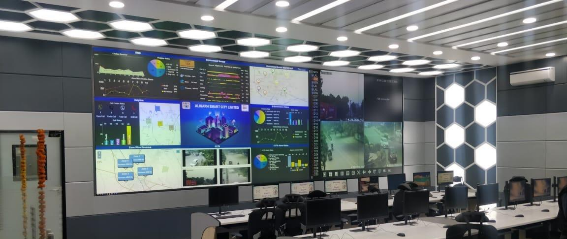
Project: Aligarh Smart City-ICCC Product Installed: 5x3 70" Laser DLP Video wall Location : Uttar Pradesh (India)
