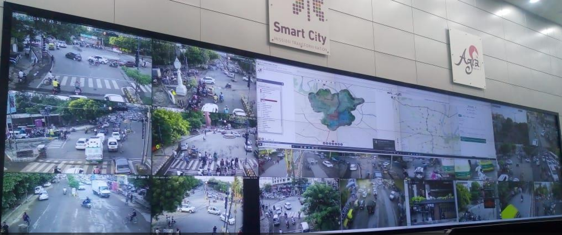
Project: Agra Smart City- ICCC Product Installed: 8x3 70" Laser DLP Video wall Location : Uttar Pradesh (India)
